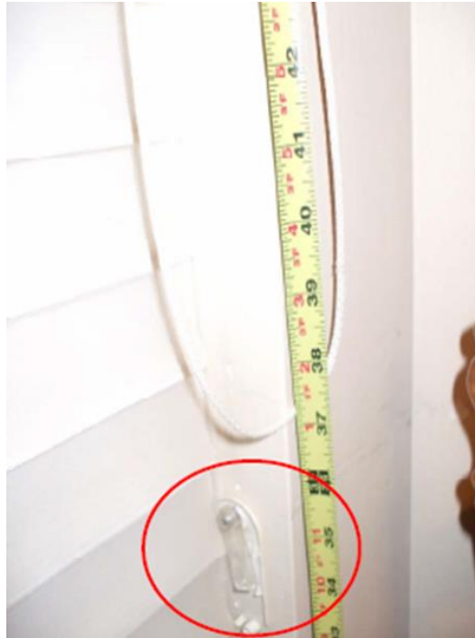
Figure 1. Broken tension device in IDI.
