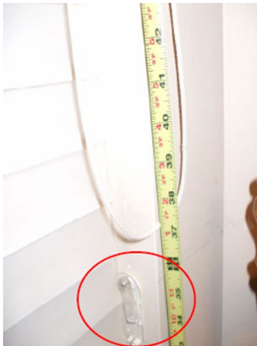
Figure 20. Broken tension device in IDI
